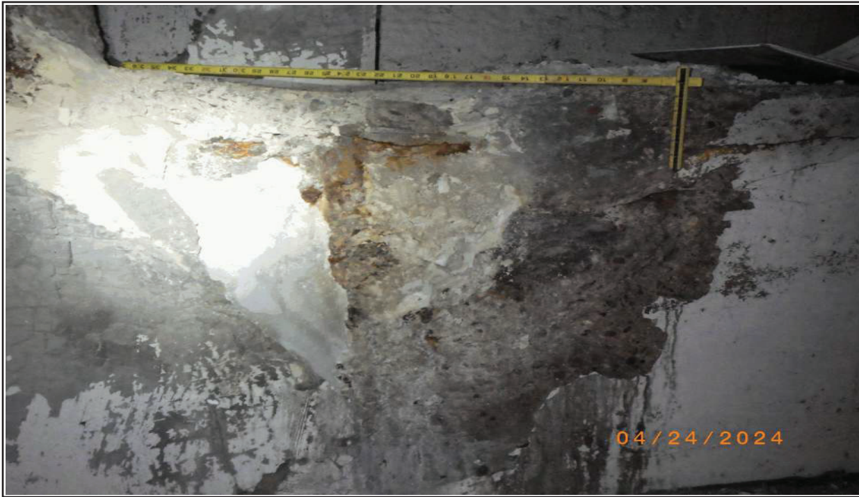
23 SPAN 3, NORTH ABUTMENT BREASTWALL BELOW BAY 5 - SPALL WITH ECSR
