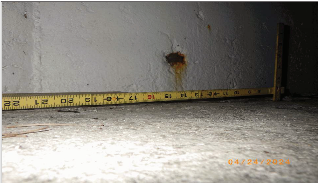
22 SPAN 3, NORTH ABUTMENT BACKWALL, WEST END - SPALL WITH ECSR AND SECTION LOSS
