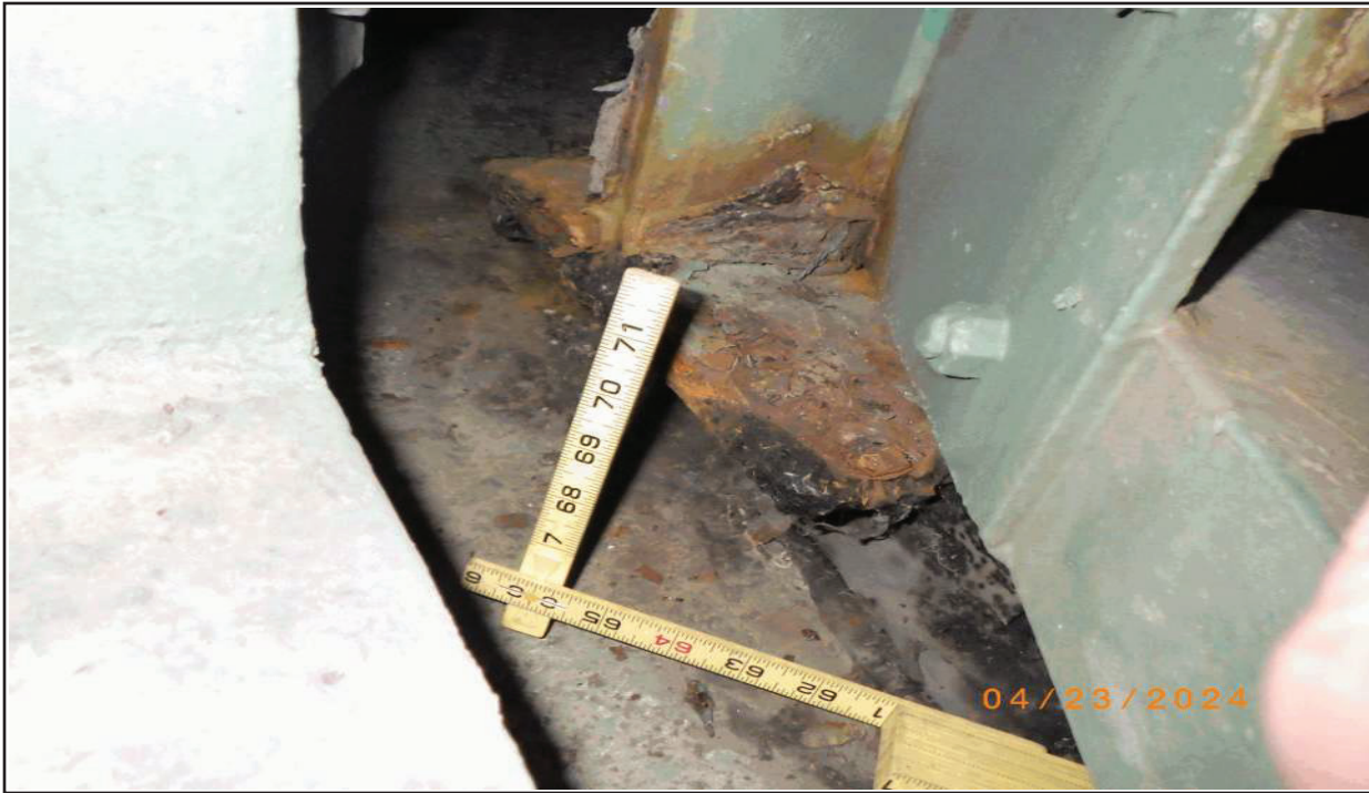
15 SPAN 2, GIRDER 5, EAST BOTTOM FLANGE AT PIER 1 - CORROSION WITH LOSS OF SECTION
