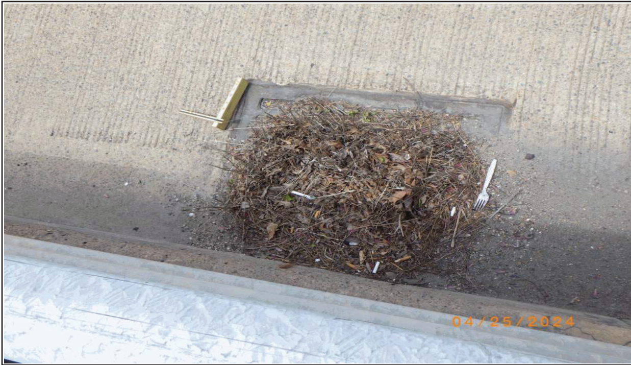
11 SPAN 3, EAST DRAIN - FULLY CLOGGED
