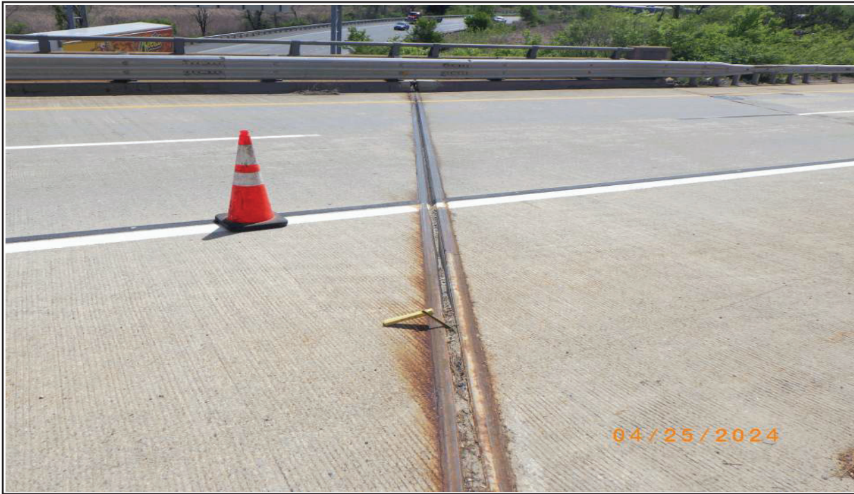
9 SPAN 1, SOUTH ABUTMENT STRIP SEAL - JOINT ARMORING HAS CORROSION WITH SECTION LOSS
