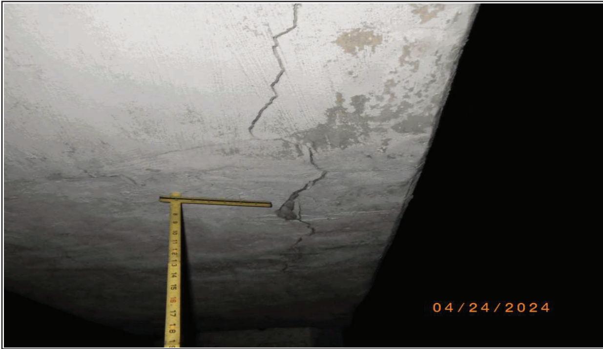
25 SPAN 2, PIER 2, UNDERSIDE OF CAP BETWEEN COLUMNS 2 AND 3 - LONGITUDINAL CRACKS
