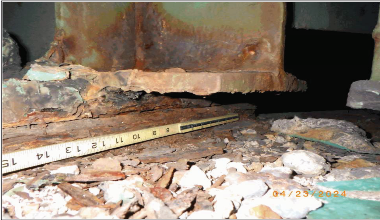
17 SPAN 1, BEARING 6 AT PIER 1, NORTH FACE - CORROSION AND LOSS OF SECTION TO MASONRY PLATE
