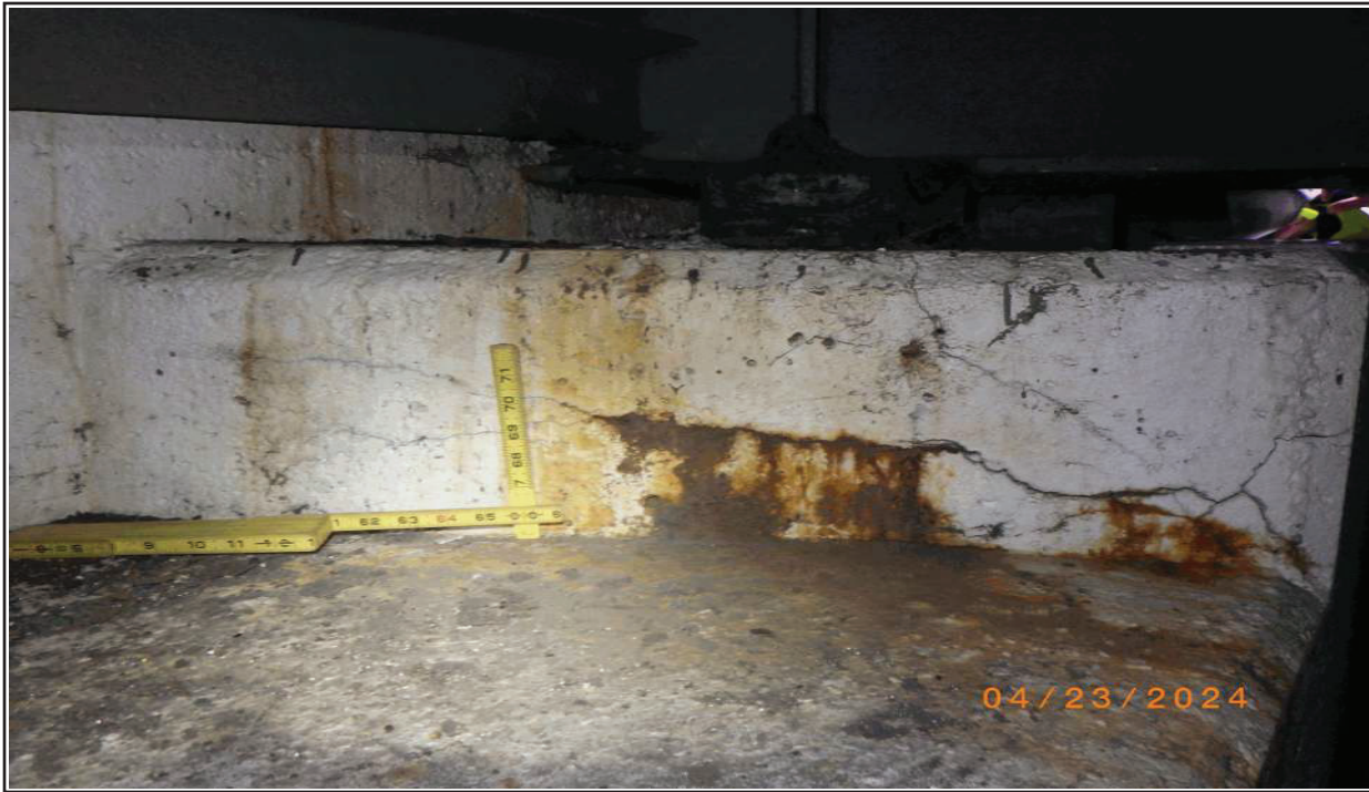
19 SPAN 1, SOUTH ABUTMENT, BEARING 5 SEAT, EAST FACE - HORIZONTAL CRACKS WITH CORROSION STAINING
