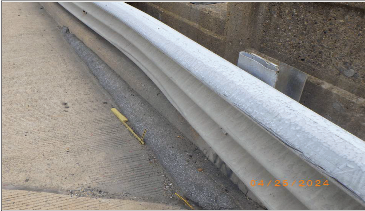
7 SPAN 1, EAST THRIE BEAM AT SOUTH ABUTMENT - IMPACT DAMAGE
