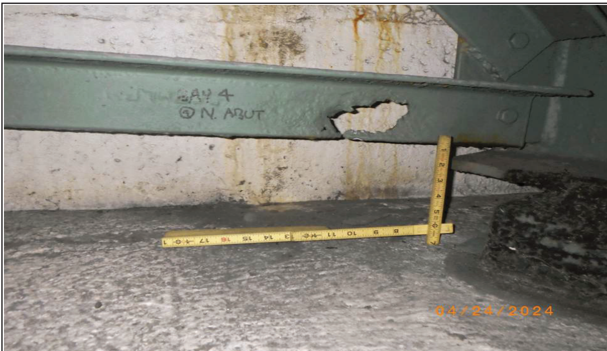
16 SPAN 3, BAY 4 DIAPHRAGM AT NORTH ABUTMENT - PAINTED OVER SECTION LOSS IN BOTTOM ANGLE
