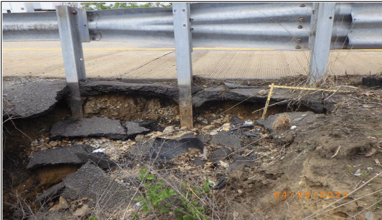
26 SOUTHEAST EMBANKMENT - EROSION BEHIND GUARDRAIL AT TRANSITION GUARDRAIL
