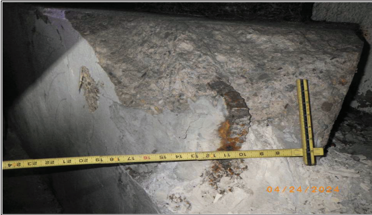
21 SPAN 3, NORTH ABUTMENT BEARING 5 SEAT BELOW BAY 5 - SPALL WITH ECSR AND SECTION LOSS
