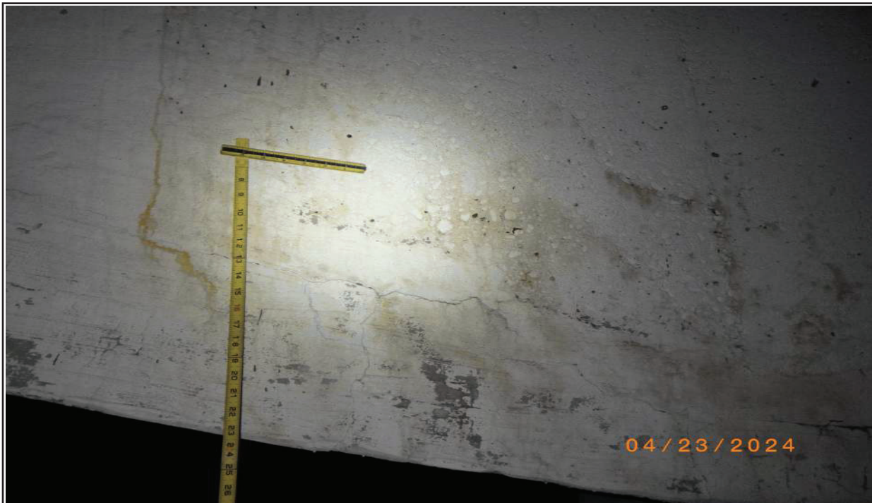
24 SPAN 1, PIER 1, SOUTH FACE OF CAP ABOVE COLUMN 3 - CRACK WITH CORROSION STAINING
