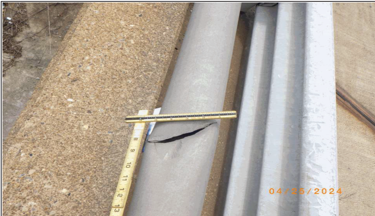
8 SPAN 1, EAST ALUMINUM RAIL BETWEEN POSTS 5 AND 6 - DISTORTION WITH CRACK
