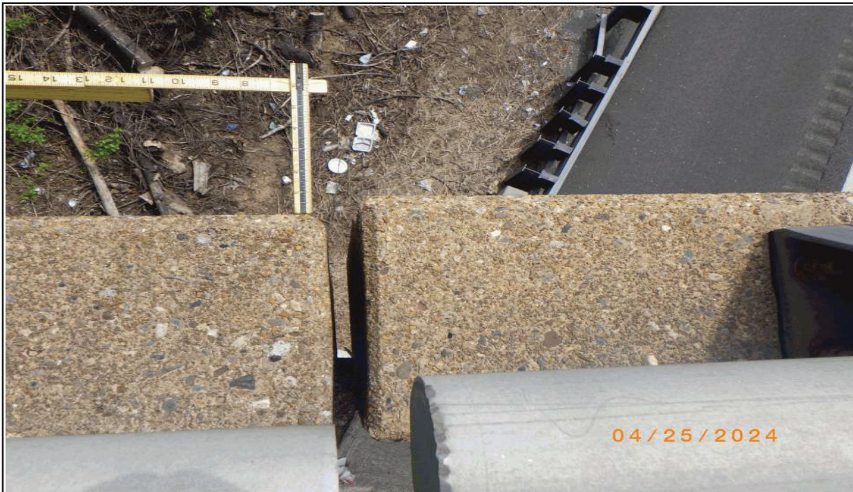
10 SPAN 2, SPAN IS HORIZONTALLY MISALIGNED TOWARDS THE EAST AT THE NORTH ABUTMENT
