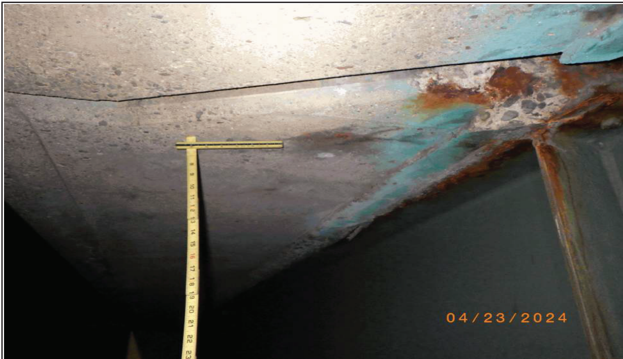
12 SPAN 1, SOFFIT IN BAY 2 AT SOUTH ABUTMENT - SPALL EXPOSING TOP FLANGE OF GIRDER
