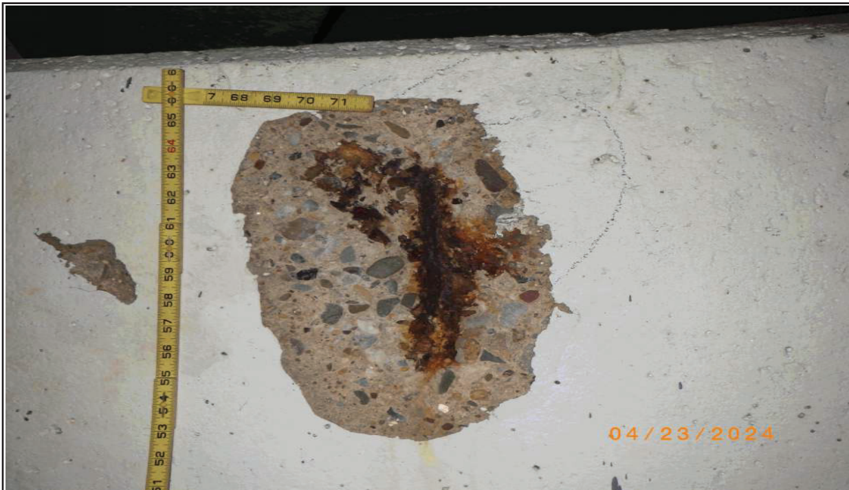
20 SPAN 1, SOUTH ABUTMENT, BREASTWALL BELOW GIRDER 6 - SPALL WITH ECSR AND SECTION LOSS
