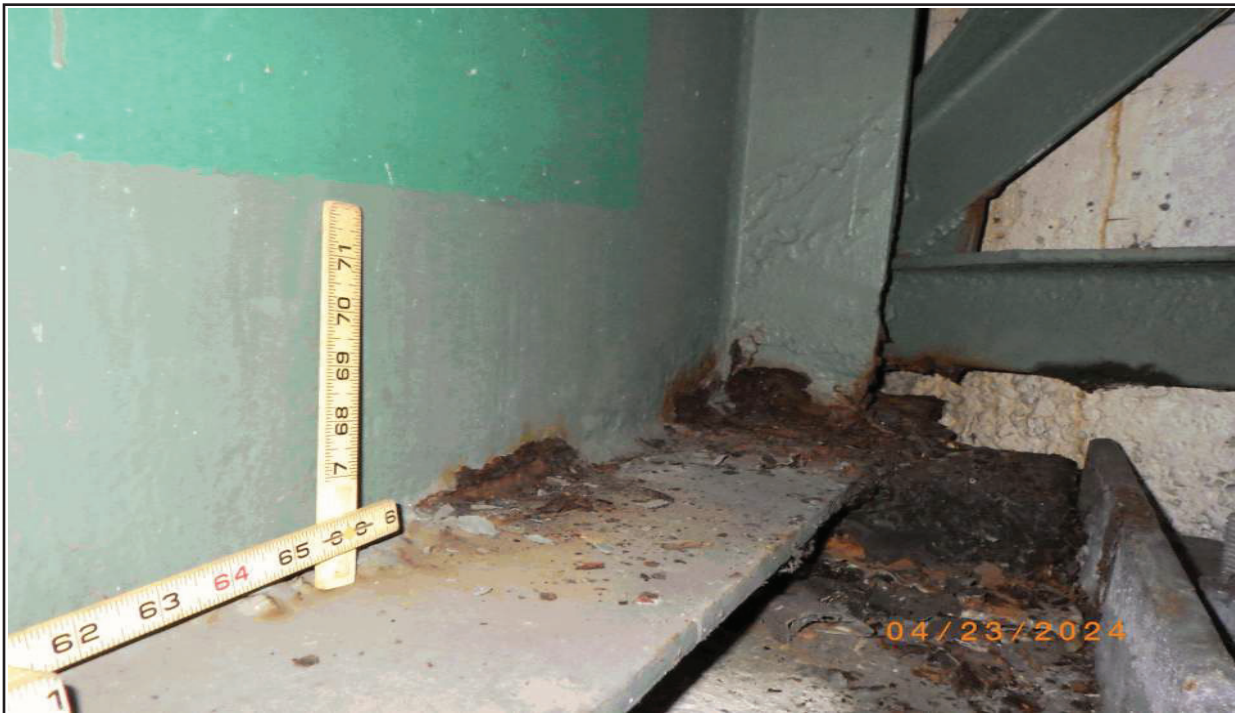
14 SPAN 1, GIRDER 5 WEST BOTTOM FLANGE AT SOUTH ABUTMENT - CORROSION WITH LOSS OF SECTION
