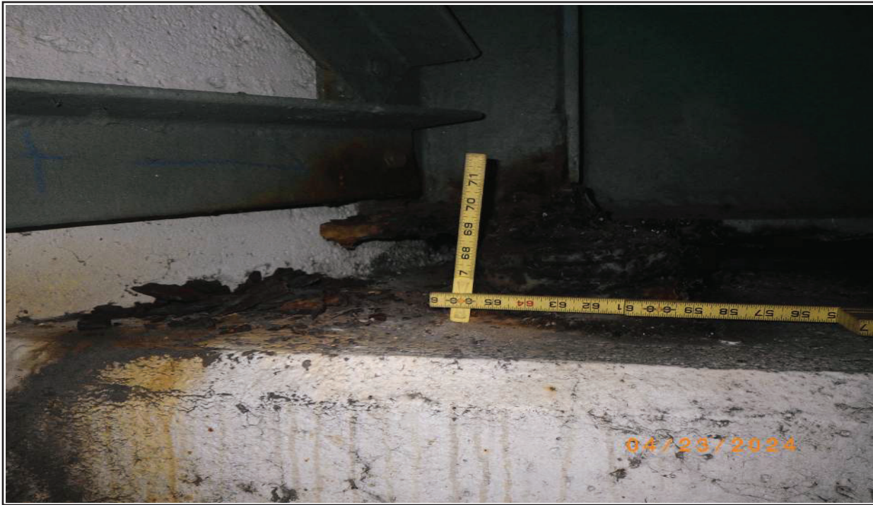
13 SPAN 1, BAY 3 END DIAPHRAGM AT SOUTH ABUTMENT - CORROSION AND PACK RUST CAUSING DISTORTION TO ANGLE
